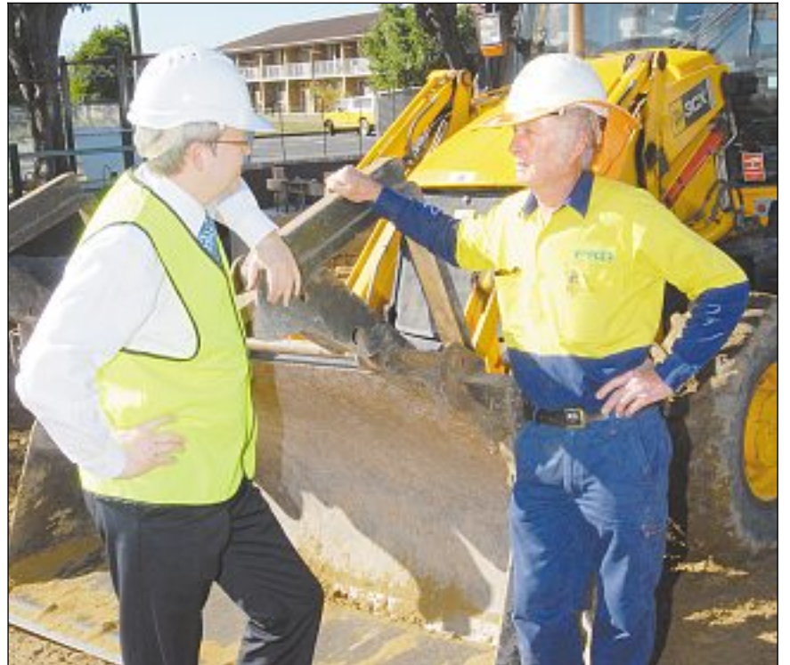
Kevin Rudd chats with FK Gardner and Sons site manager Colin Feeney at the Central State School building site yesterday. PHOTO: PETER HOLT 230709/087
